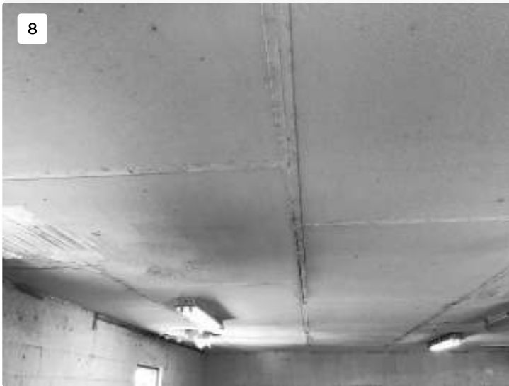
Project: SA-23-2007-REP (DKI) Date: 6/6/2023, 1:59pm Creator: Robert Patton Tags: utility room
