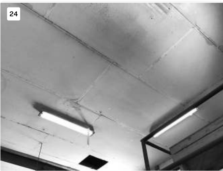
Project: SA-23-2007-REP (DKI) Date: 6/6/2023, 2:01pm Creator: Robert Patton Tags: utility room
