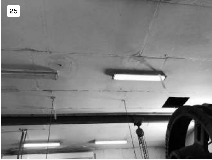
Project: SA-23-2007-REP (DKI) Date: 6/6/2023, 2:01pm Creator: Robert Patton Tags: utility room
